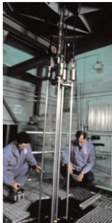
Coolant Water Filtration at a Nuclear Plant
