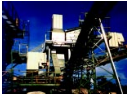
Screening and conveying
