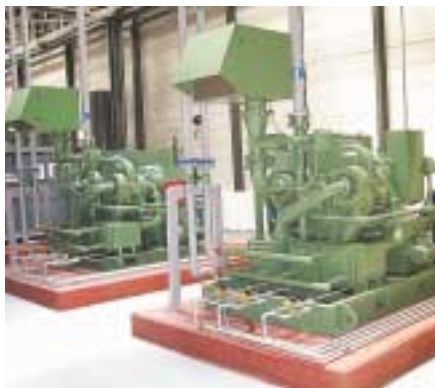
350 HP (260 kW) Turbo Air® Compressors installed at an automotive facility.
