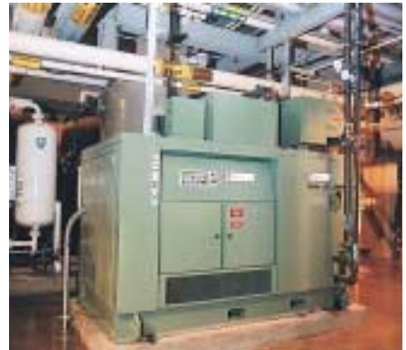
One 300 HP (225 kW) Turbo Air® Compressor installed at a major university for instrument air.
