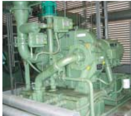
300 HP (225 kW) Turbo Air® Compressor installed at a semiconductor facility.
